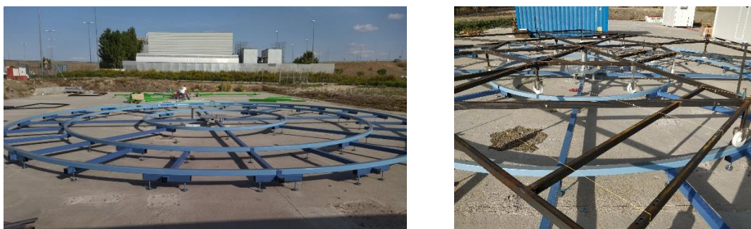
Fig. 3. Installed rail-paths of the SunDial (left); and rotatory platform of the SunDial installed on top of the rail-paths (right).
