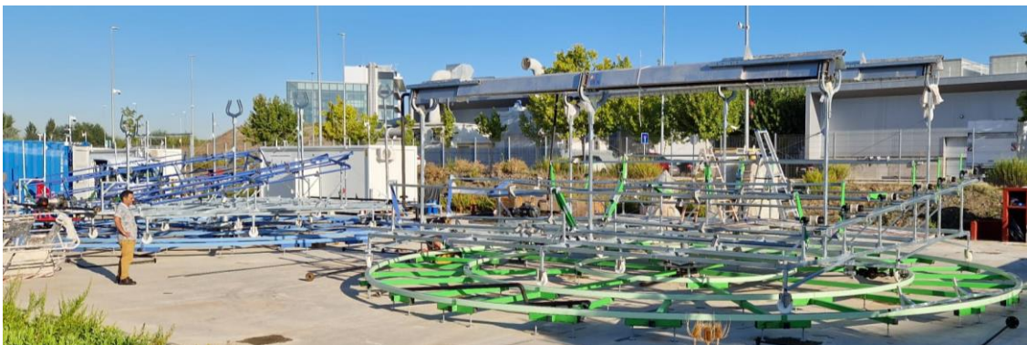
Fig. 8. Present state of the installation.
